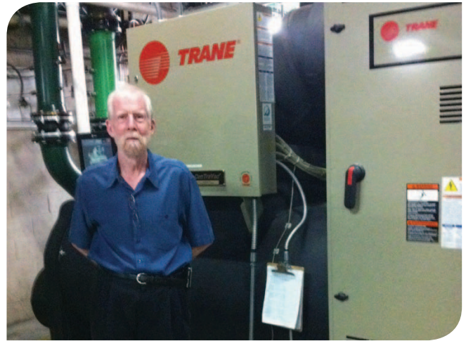
With three Trane CenTraVac centrifugal chillers and Tracer Summit BAS, Pat Ware, chief engineer, Four Seasons Resort Maui, optimizes central plant operations to reduce energy consumption.
